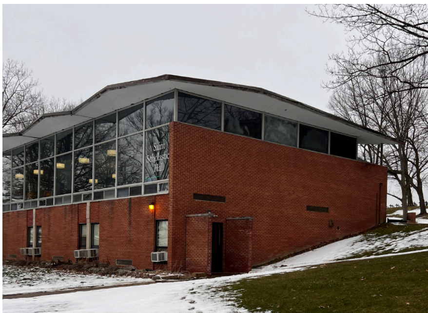
Saint Scholastica Hall suffered damage to its roof during a storm. (SOURCE: ADOMAITIS)
